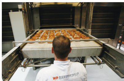
WP Matador oven and automatic loader
